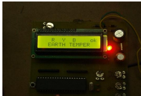
Earth fault Detected
