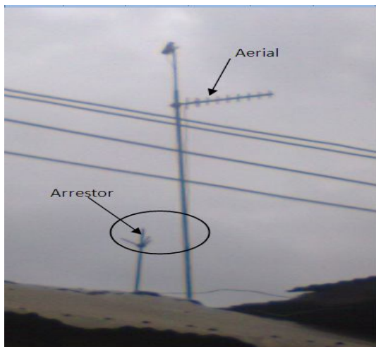
Figure 4: Common Lightning rod installation (wrong Positioning)
